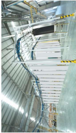
Spraying Line (German WAGNER Spraying Room)
